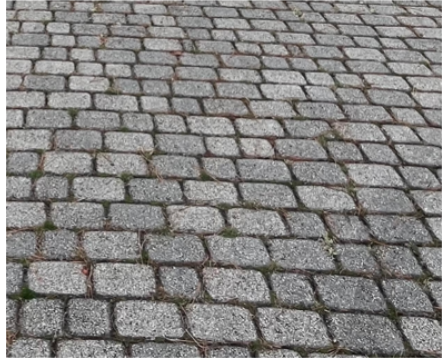
DRIVEWAY PAVERS MANUFACTURE: UNKNOWN, EXISTING TO REMAIN COLOR: GRAY INSTALLATION: SET ON SAND
