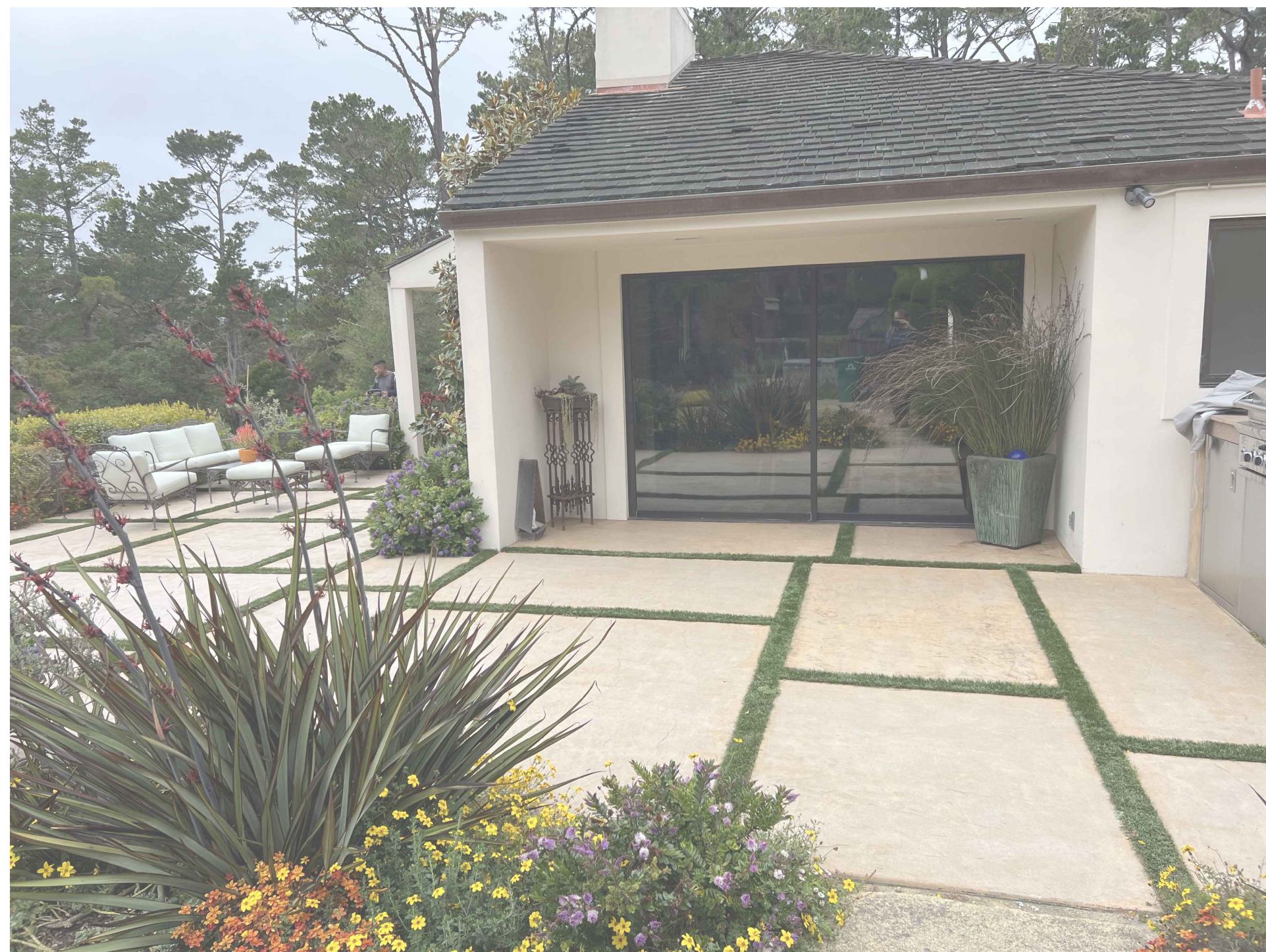
3 EXISTING PHOTOGRAPH LOOKING NORTHWEST AT EXISTING EXTERIOR SIDE OF KITCHEN TO BE RENOVATED WITH NEW ADDITION
