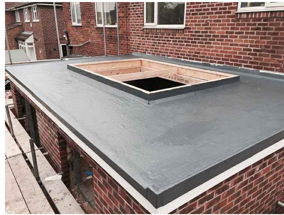
RUBBER MEMBRANE ROOF SYSTEM WHITE OR LIGHT COLOR WITH HIGH ALBEDO / HIGH EMISSIVITY
