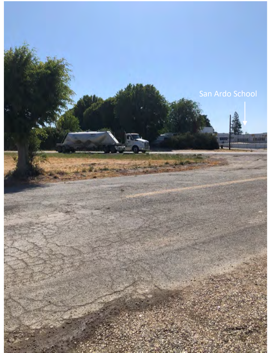
Intersection of Godchaux Street and Cattlemen Road Proposed improvements to this intersection include crosswalk and pedestrian beacons
