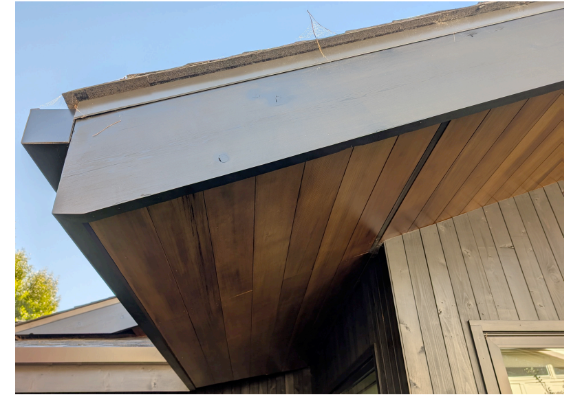
Eaves Painted Metal Gutters - Black to Match Main Residence Painted Cedar Fascia Board - Black to Match Main Residence Stained 1x6 Cedar Soffit to Match Main Residence with 1/2" Densdeck Class 'A' Underlayment
