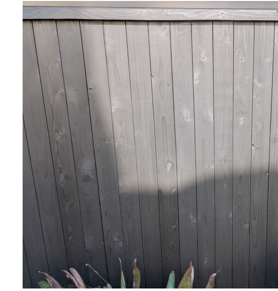
Siding Vertical 1x4 T&G Cedar Siding Painted - Black with 1/2" Densdeck Class 'A' Underlayment
