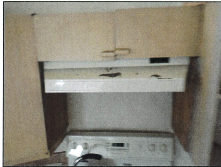
Damaged vent noted.
