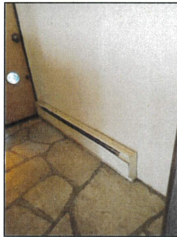
Unit did not appear to operate.
