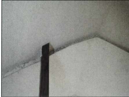
Indications of moisture and fungus growth,
