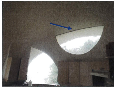
Staining at top window line noted.
