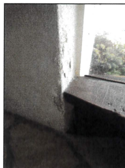
Window failure has cause to water damage.
