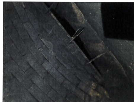
Deteriorated damper noted.
