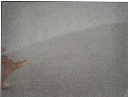
Water stains noted throughout the home.
