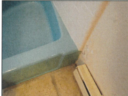
Water damage noted
