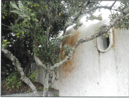
Areas of hollow sounding and potentially detached stucco noted.
