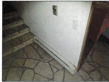
Thermostat found above heater.
