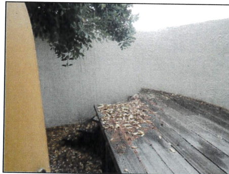
Areas of water damage at wall to deck connection.
