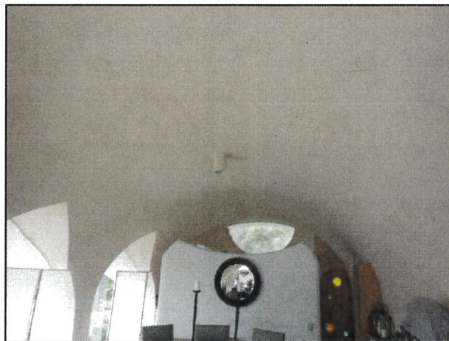
Areas of water staining noted.
