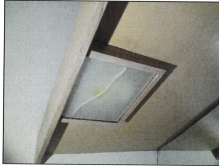
Broken cover plate.
