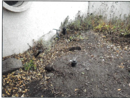
Areas of repairs noted.
