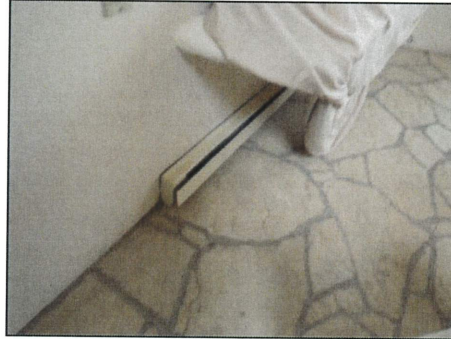
Heater found rusted. Most did not operate when tested.
