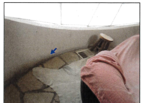
Extensive water staining at floor line.
