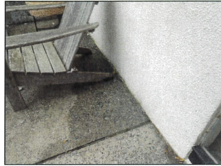
No weep screed was found.
