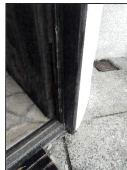
Areas of deteriorated jambs.
