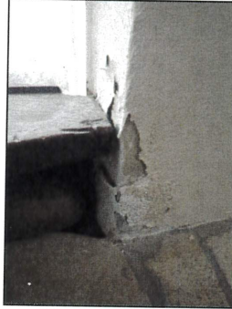
Extensive water damage noted.
