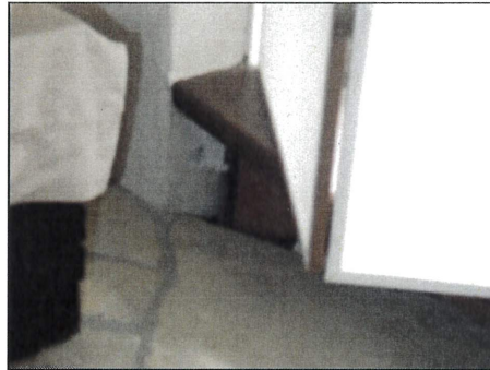
Areas of water damage noted.
