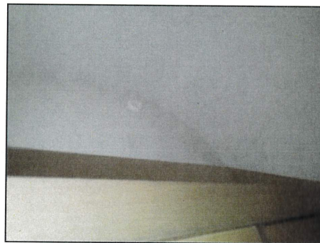
Missing detector noted.
