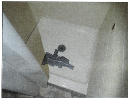
Large cracked shower pan noted.
