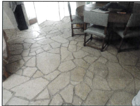
Floors are uneven and present a tripping hazard.
