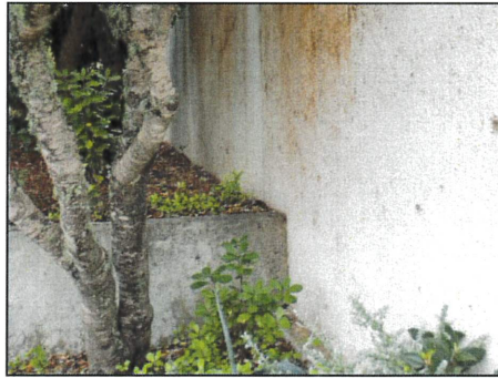
Potential areas of water damage at planter.
