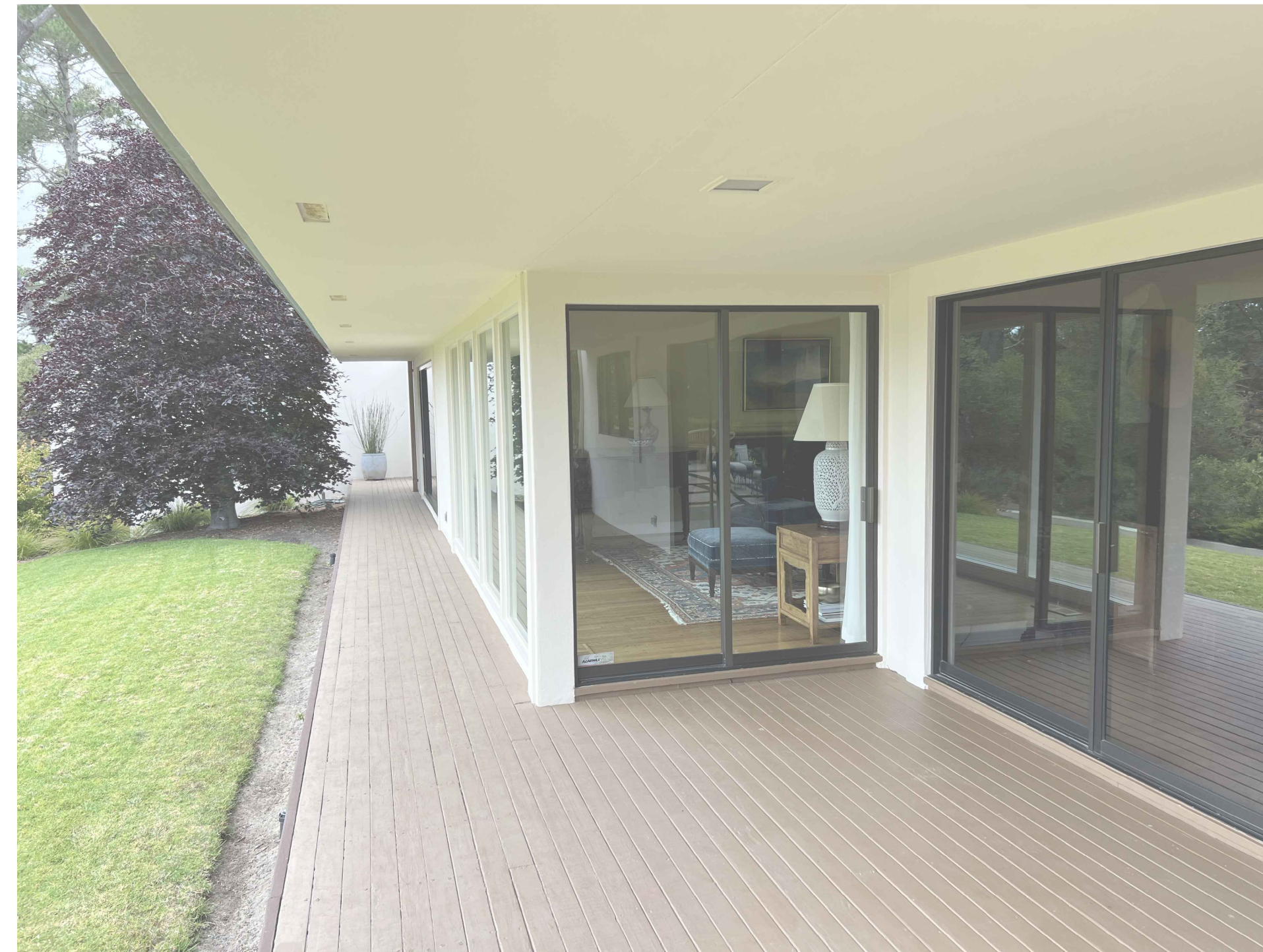
5 EXISTING PHOTOGRAPH LOOKING NORTHWEST AT EXISTING DECK; AREA SHOWN TO REMAIN, NO CHANGE
