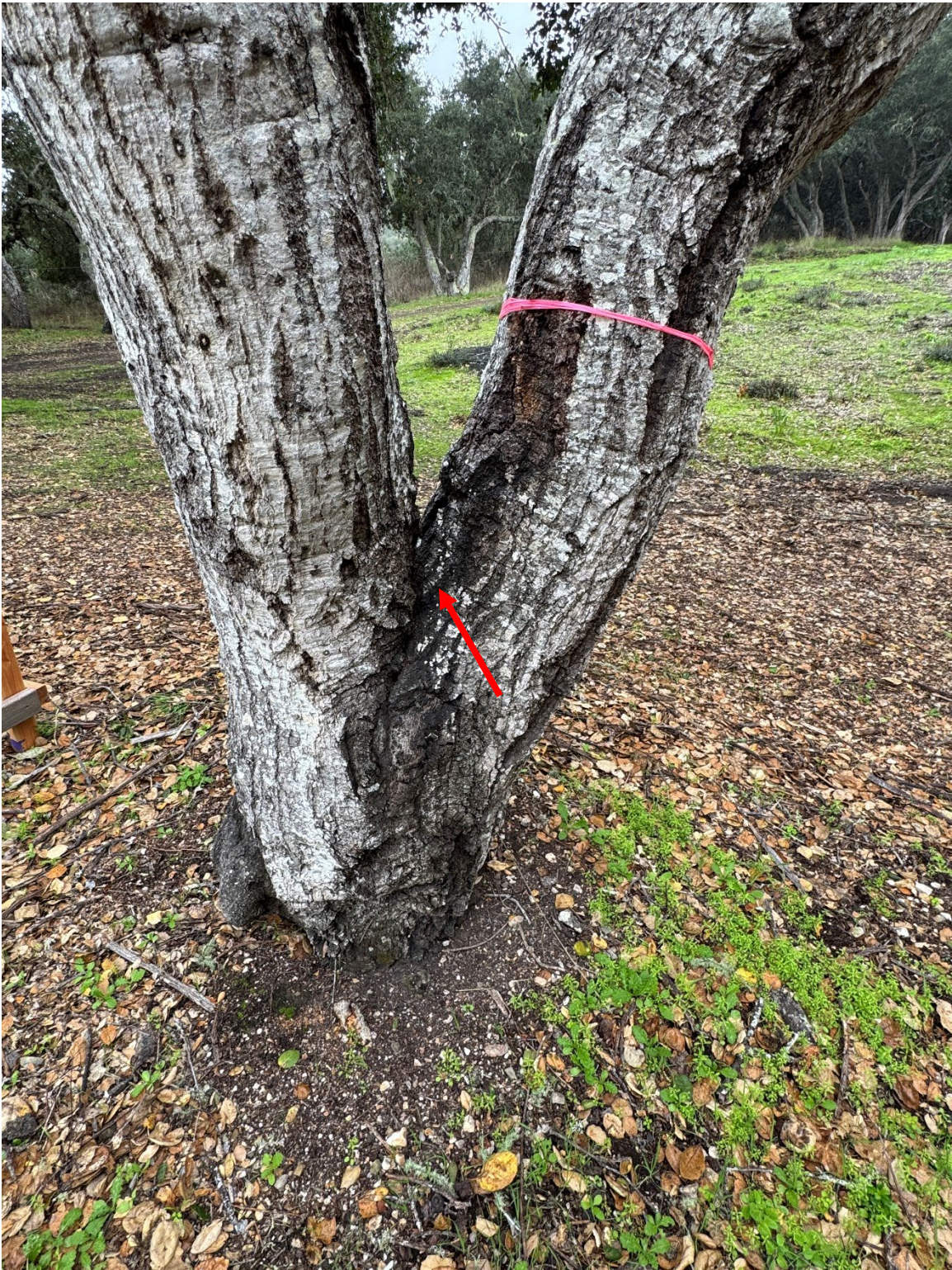
Tree #966 with structurally weak branch attachments, decay in stem, and multiple beetle attacks.
