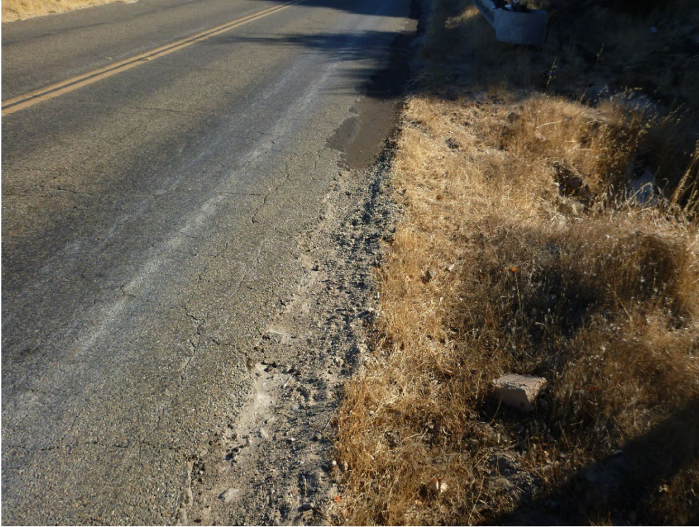
2019 Photograph 13. Erosion along inside edge of roadway. Note minor cracks and asphalt patch in upper middle.
