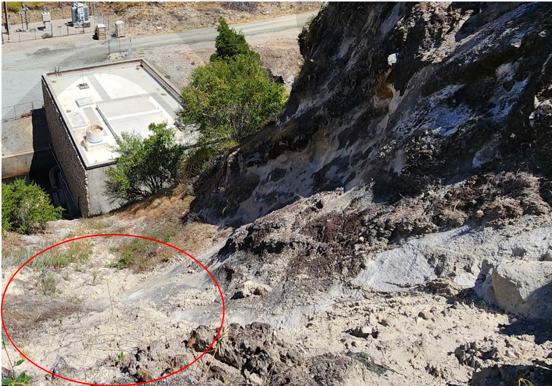
2024 Photograph 2. Minimal change from 2019. Veneer of new colluvial debris in lower left (circled).
