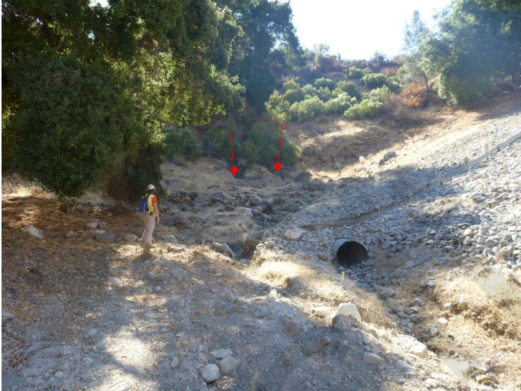
2019 Photograph 23. Gullies on slopes above right downstream groin of dam. The arrows mark the downstream end of the gully shown in Photograph 22.
