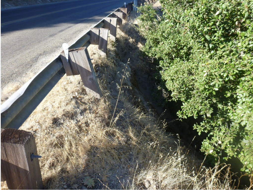
2019 Photograph 21. Guardrail post undermined at head of gully above culvert outfall.
