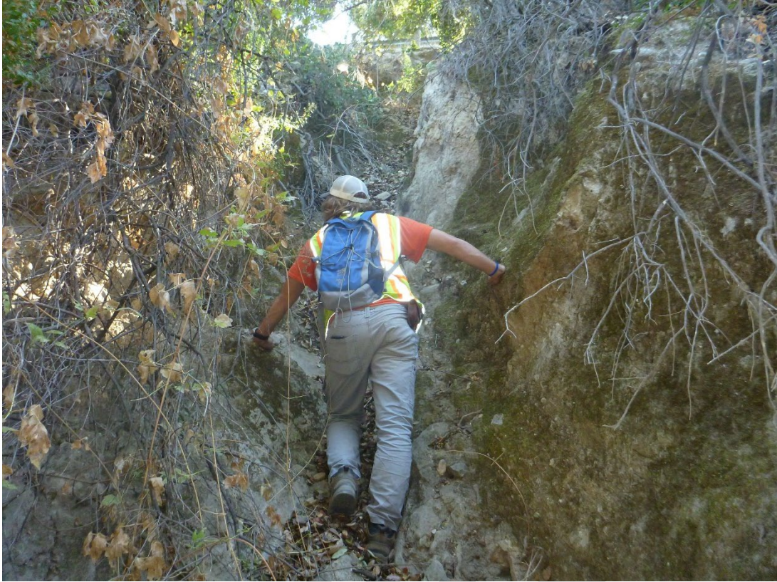
2019 Photograph 22. Deep erosion gully below culvert. Note guardrail in top middle of photograph.
