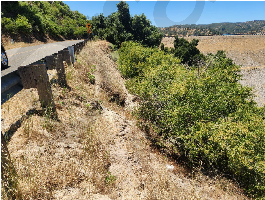
2024 Photograph 18. Continued shallow sloughing of upper fill slopes.
