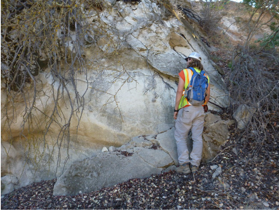
2019 Photograph 6. Failed slab of rock. Note roots on failure surface and in fractures in front of the geologist.
