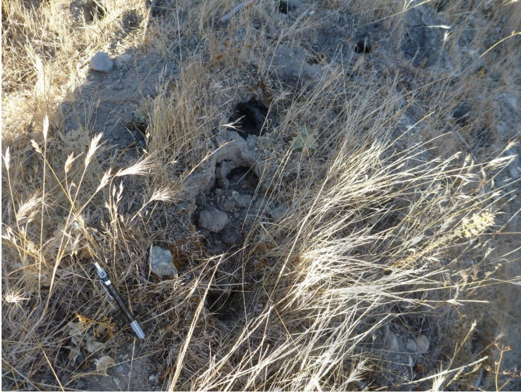
Photograph 19. Network of burrows in loose, sandy fill at edge of road.
