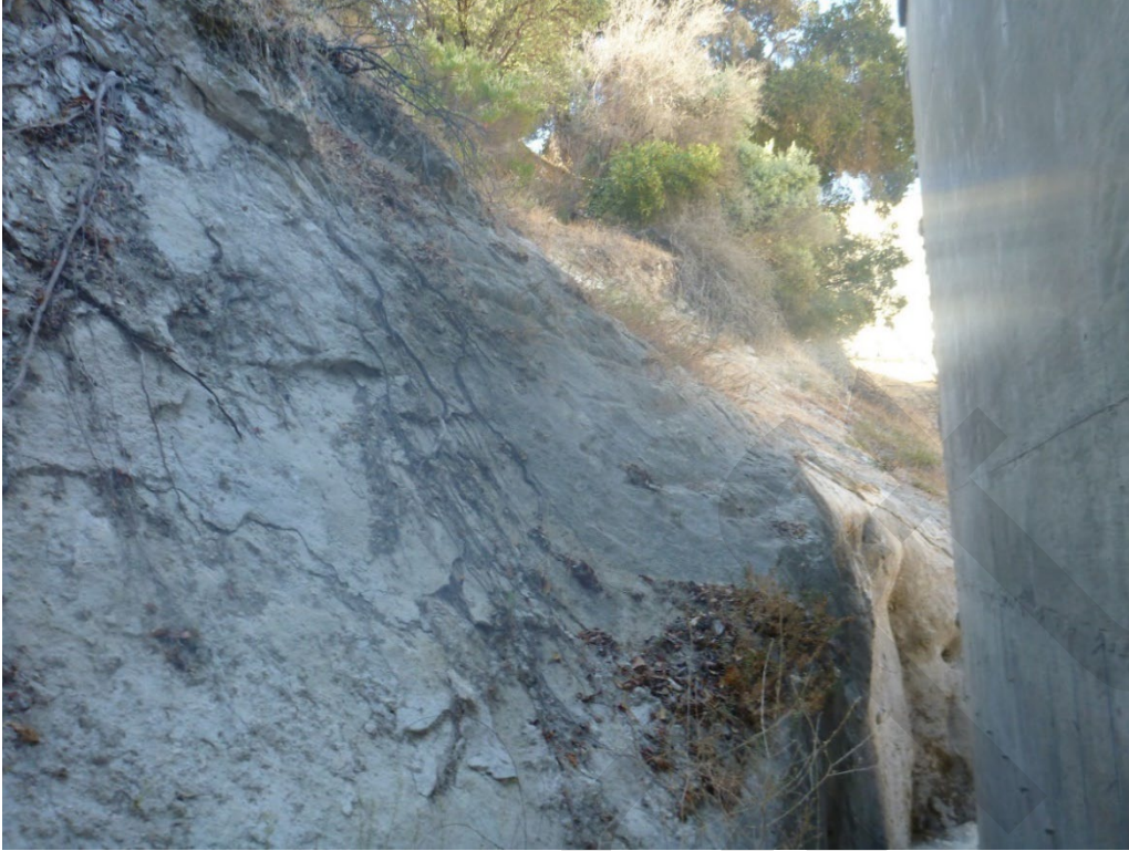
Photograph 8. Failed slab of rock behind Powerhouse. Note roots on the failure surface.
