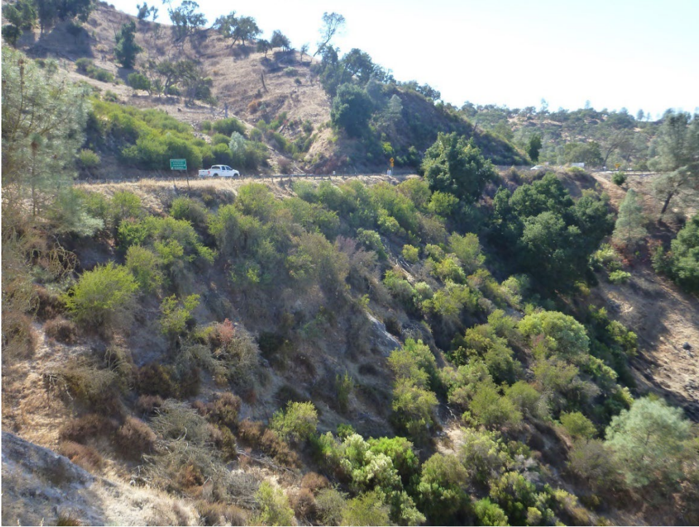
2019 Photograph 11. Lake Nacimiento Drive, showing cuts above road and fills below.
