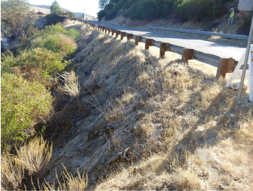
2019 Photograph 17. Shallow sloughing of upper fill slopes (looking east).
