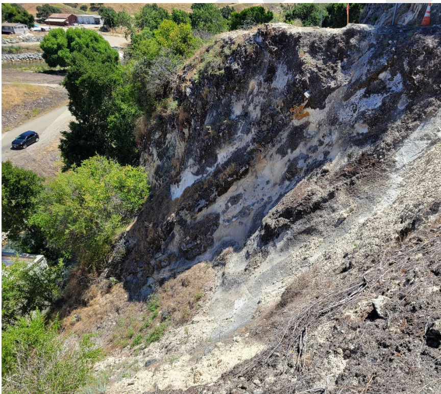
2024 Photograph 10. Veneer of new colluvial debris since 2019.
