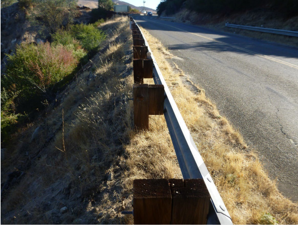
2019 Photograph 16. Same area shown in Photograph 15. Note straight guardrail and plumb posts.
