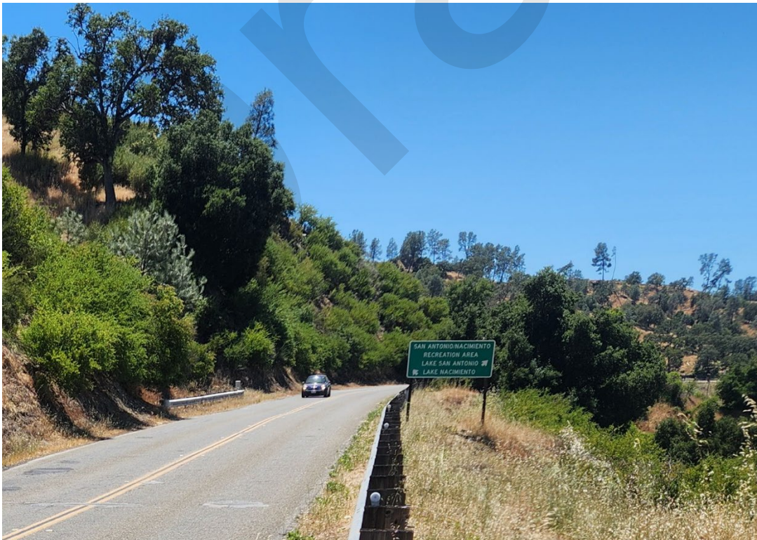
2024 Photograph 12. Minor road patch repairs since 2019. Marginal difference in overall road condition.
