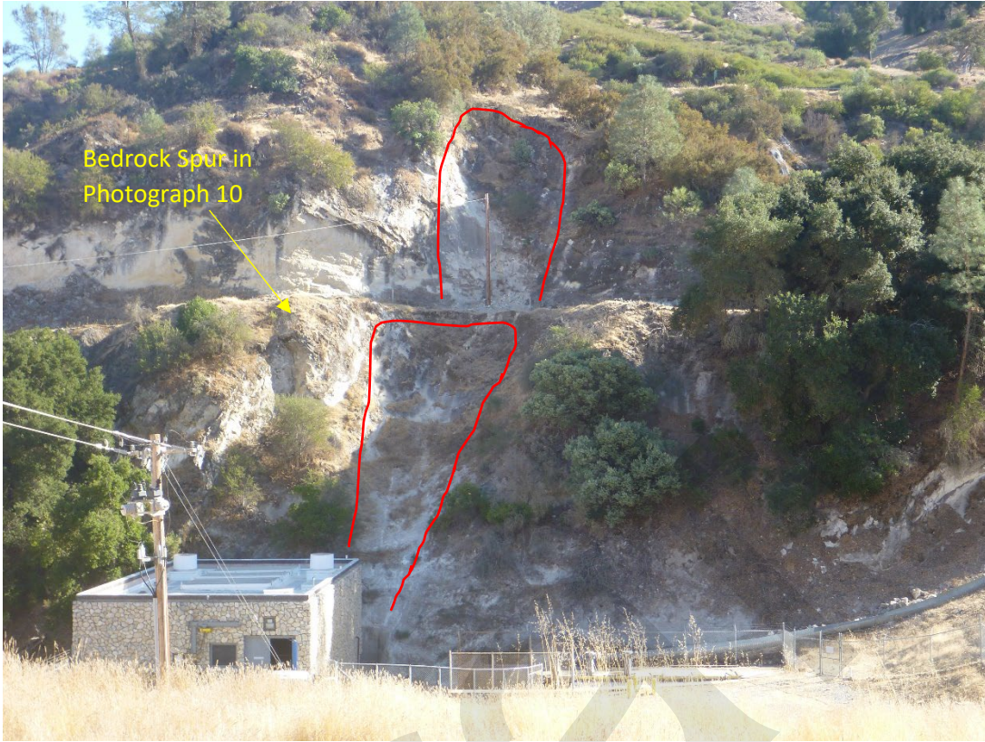
2019 Photograph 1. Slopes above Nacimiento Powerhouse showing the swale (red lines) that failed in 1995.
