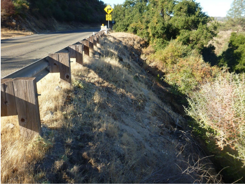
2019 Photograph 18. Shallow sloughing of upper fill slopes (looking west).
