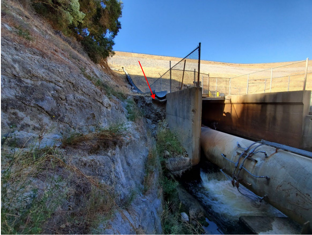
2019 Photograph 3. Cut slope at bottom of swale and exposed penstock. Note half-round CMP and erosion of wall backfill.
