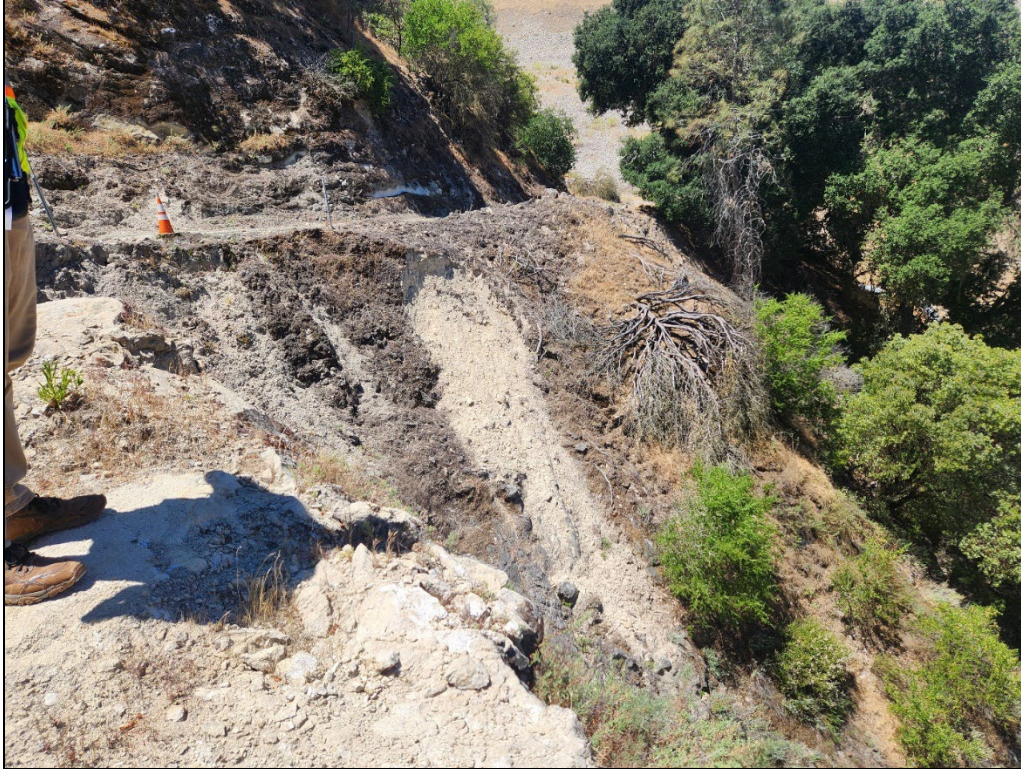
Photograph 2024-2. Recent shallow failure above Powerhouse and erosion along edge of access road. View is to the West.
