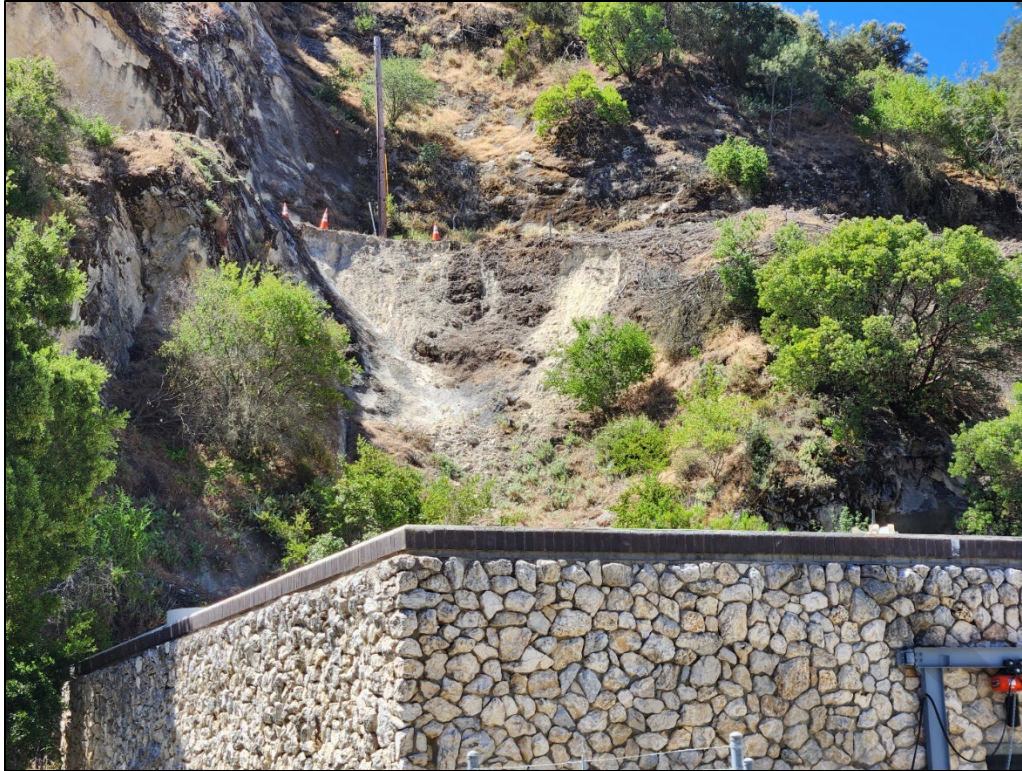
Photograph 2024-4. View of the recent shallow failure and erosion along the edge of the access road from below. View is to the South.
