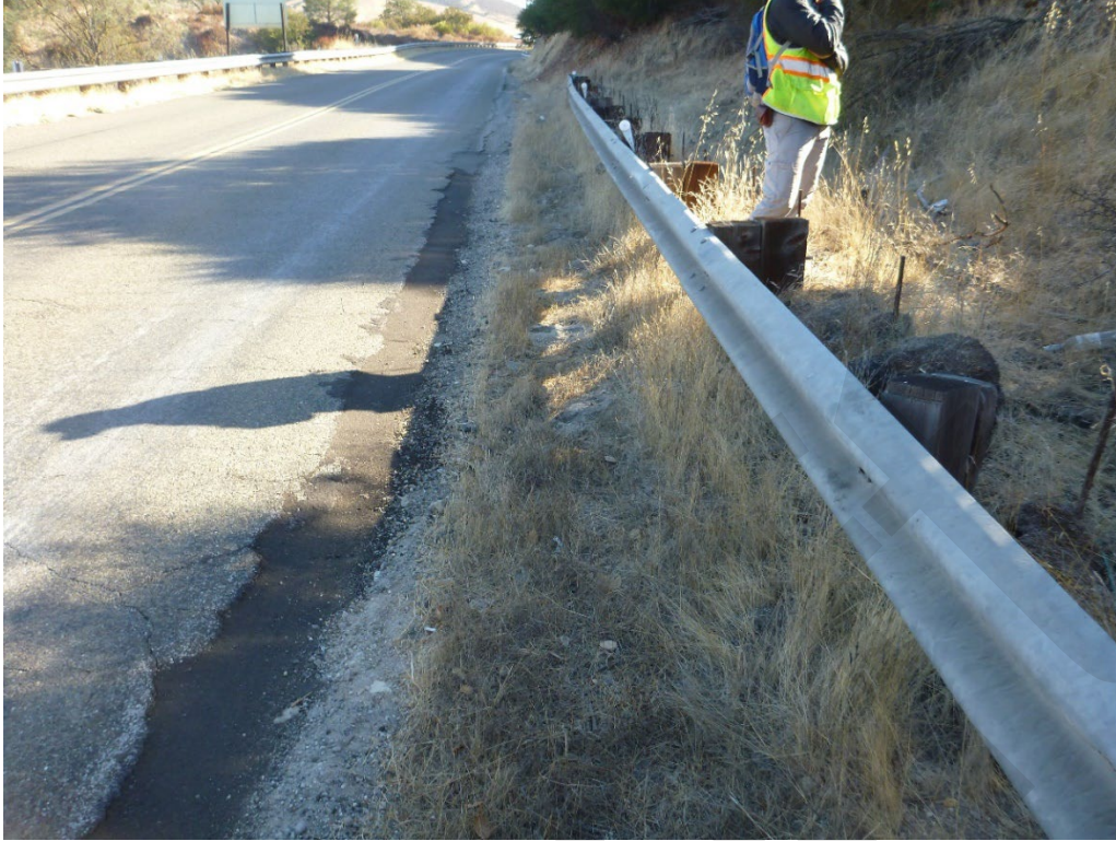
2019 Photograph 14. Asphalt patch in area of erosion along inside edge of road.
