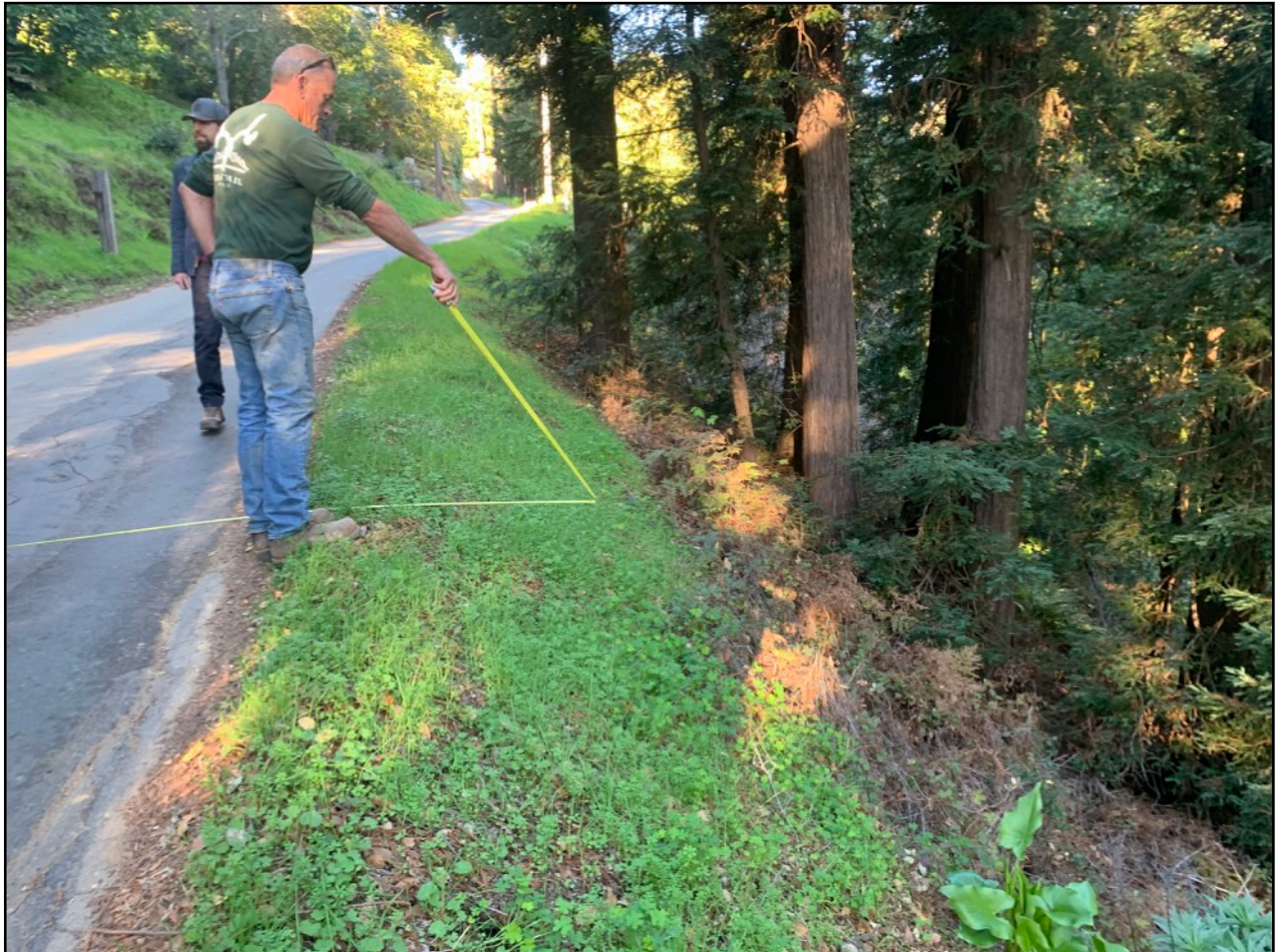
Road edge ruderal vegetation with tape measure showing the extent of the limits of grading that will be required for excavation to install the hilfiker system.
